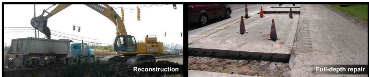
Figure 3: Examples of reconstruction treatments—(left) reconstructing a road and (right) road prepared for full-depth repair.
