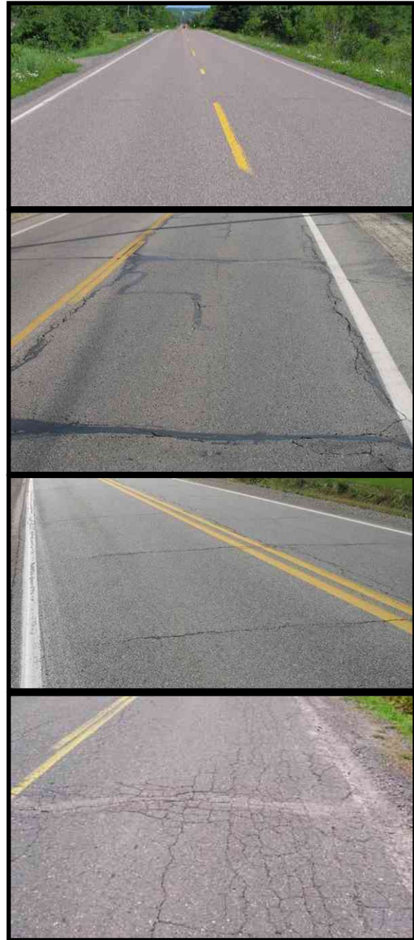
Figure 1: Top image, right – PASER 8 road that is considered “good” by the TAMC exhibit only minor defects. Second image, right – PASER 5 road that is considered “fair” by the TAMC. Exhibiting structural soundness but could benefit from CPM. Third image, right – PASER 6 road that is considered “fair” by the TAMC. Bottom image, right – PASER 2 road that is considered “poor” by the TAMC exhibiting significant structural distress.
